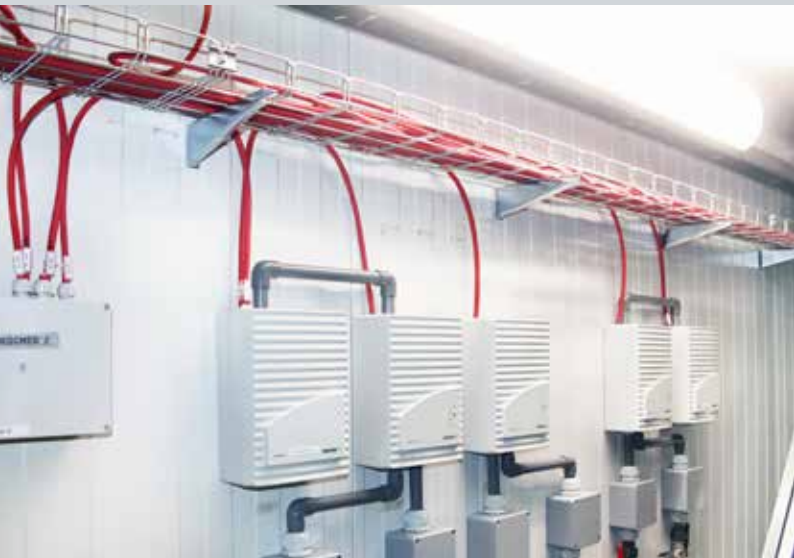
TITANUS® aspirating smoke detection systems (image above) monitor the areas protected by OxyReduct® (image on the right)
