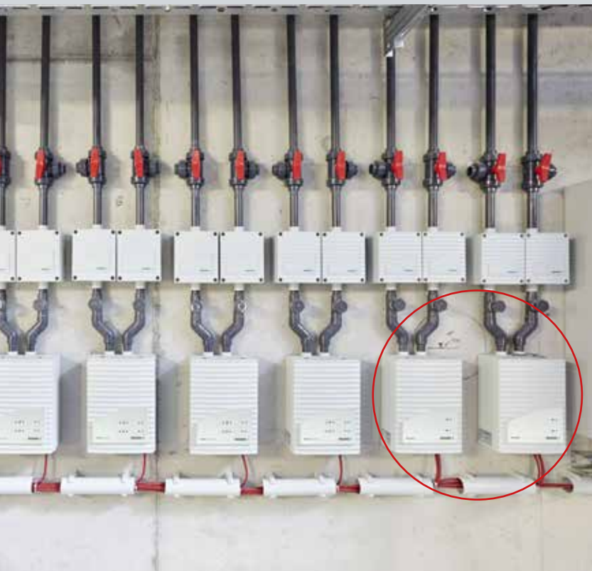
The TITANUS® system’s air sampling smoke detectors (19 units in total) were installed in a row with the OxyReduct® system’s oxygen sensors (circled in red). This means that maintenance can be conducted from a convenient central location.
