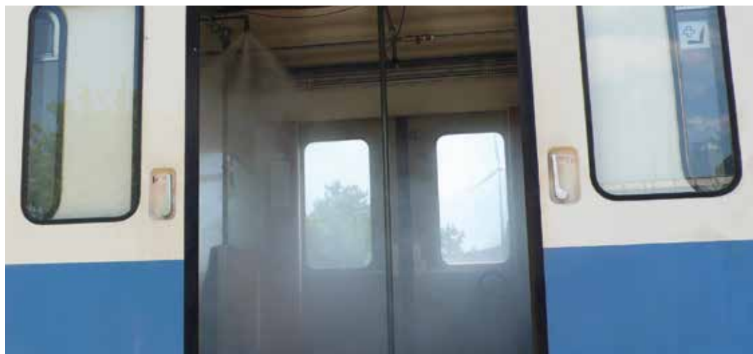
Triggered water mist system distributing fine mist spray in the passenger area.
