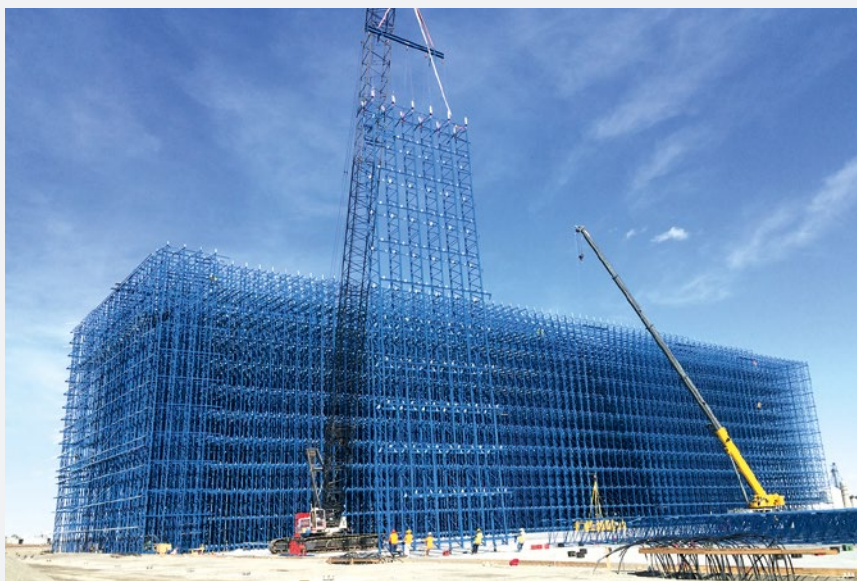
▲ Warehouses with the size and construction height of Preferred Freezer Services's represent a real challenge in terms of fire protection.
