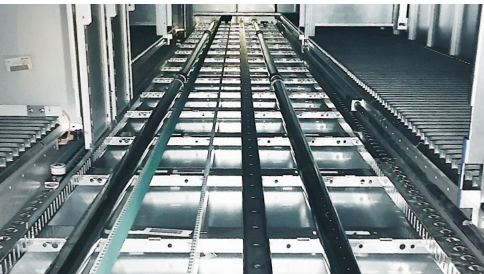
▲ View from below: Inside the approximately 12-metre warehouse lifts, diffuser pipes distribute the extinguishing gas homogeneously throughout the shuttle cab.
