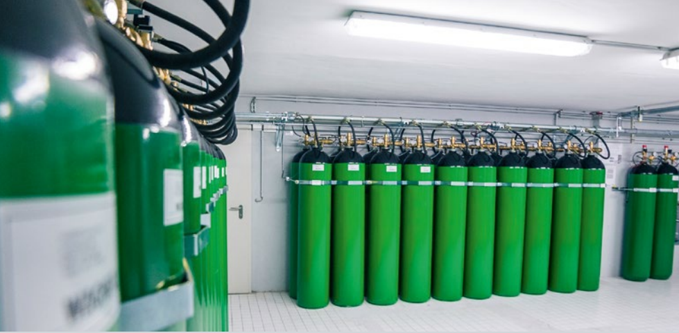
▲ The nitrogen needed to suppress any potential fires is stored in cylinder banks, from where it is directed into the data centre using a soft-flooding system using little pressure.
