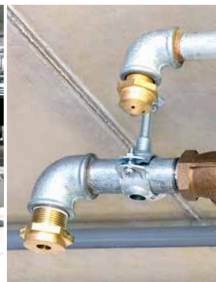
▼ The new two-stage concept combines gas extinguishing (small pipe) and oxygen reduction (large pipe).
