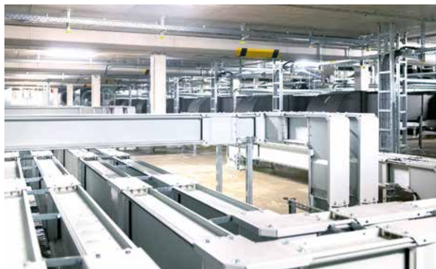
▼ Worth protecting: the two supply corridors primarily house AC and power supply lines to the data centre.
