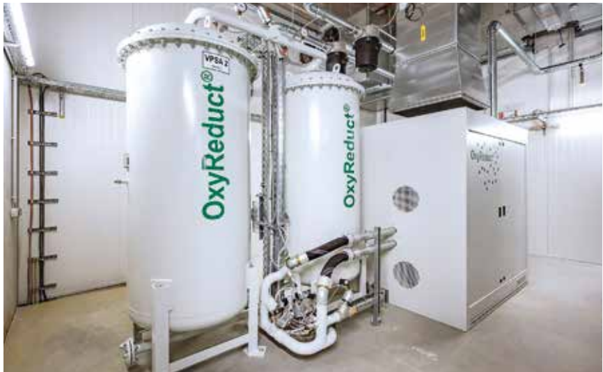
▲ The OxyReduct® system reduces the oxygen concentration level below the ignition thresholds of the main materials in the warehouse.
