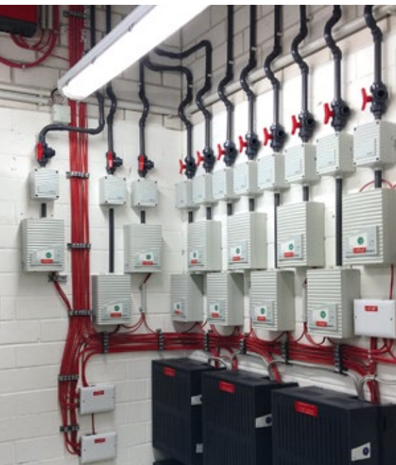
▲ The TITANUS® systems: invisible in public areas, clearly installed in the plant room.
