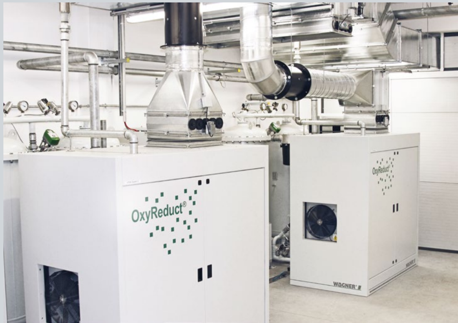
▲ OxyReduct® VPSA protects the high-bay warehouse and goods stored from the effects of fire
