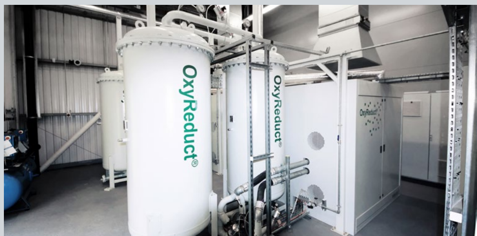
▲ Four OxyReduct® VPSA systems are installed in the Newspaper Storage Building. These generate nitrogen to reduce the oxygen content of the air within the warehouse
