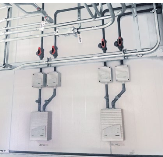
▲ The OXY-SENS® oxygen sensors are connected to the air sampling duct network
