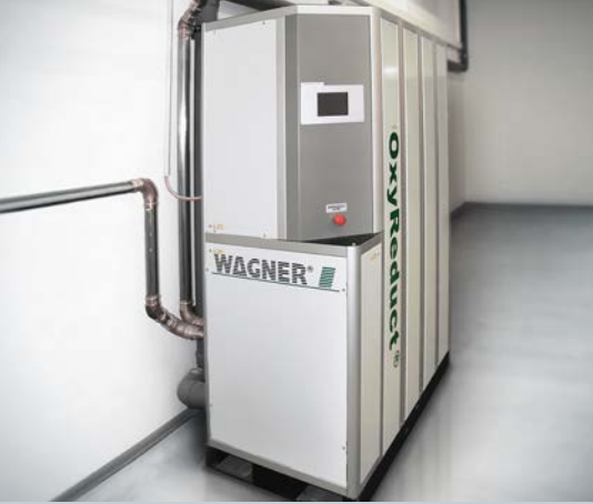
▲ The necessary oxygen reduction inside the NBG6 is achieved by an OxyReduct® fire prevention system
