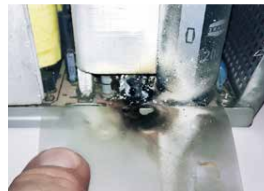
▲ A capacitor in a teleprompter began to smoulder. The part is no larger than a thumbnail, but could have destroyed the entire equipment room, had it gone unnoticed
