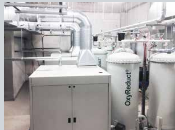
▲ Three VPSA systems with a nitrogen output of approx. 240 m³/h each were installed in KLM’s deep-freeze warehouse. One is a redundant back-up system, as required by the emergency concept
